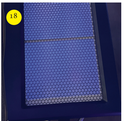
18 Check to be sure lights are illuminated when power is turned on.
